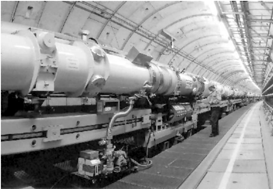
Fig. 3.3 View of the HERA tunnel [84]. The superconducting magnets of the proton storage ring are mounted above the conventional magnets of the electron ring.
