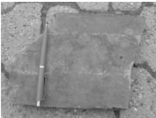
Dirty roof tile
